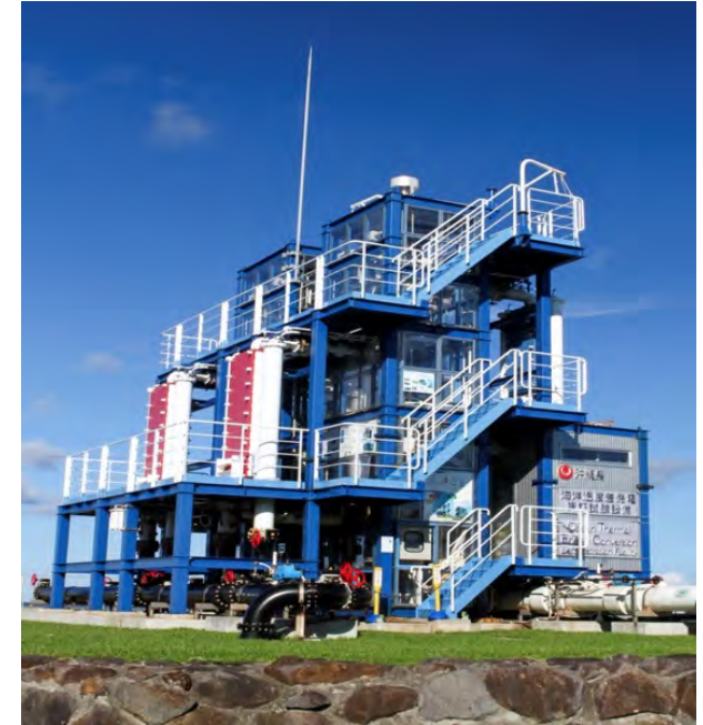
Fig.2. 50 kW OTEC plant on Kume-Island [2].
